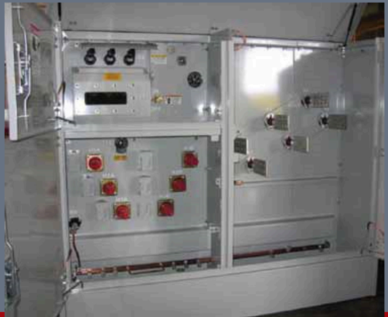
Above: Inside view of visible break transformer
